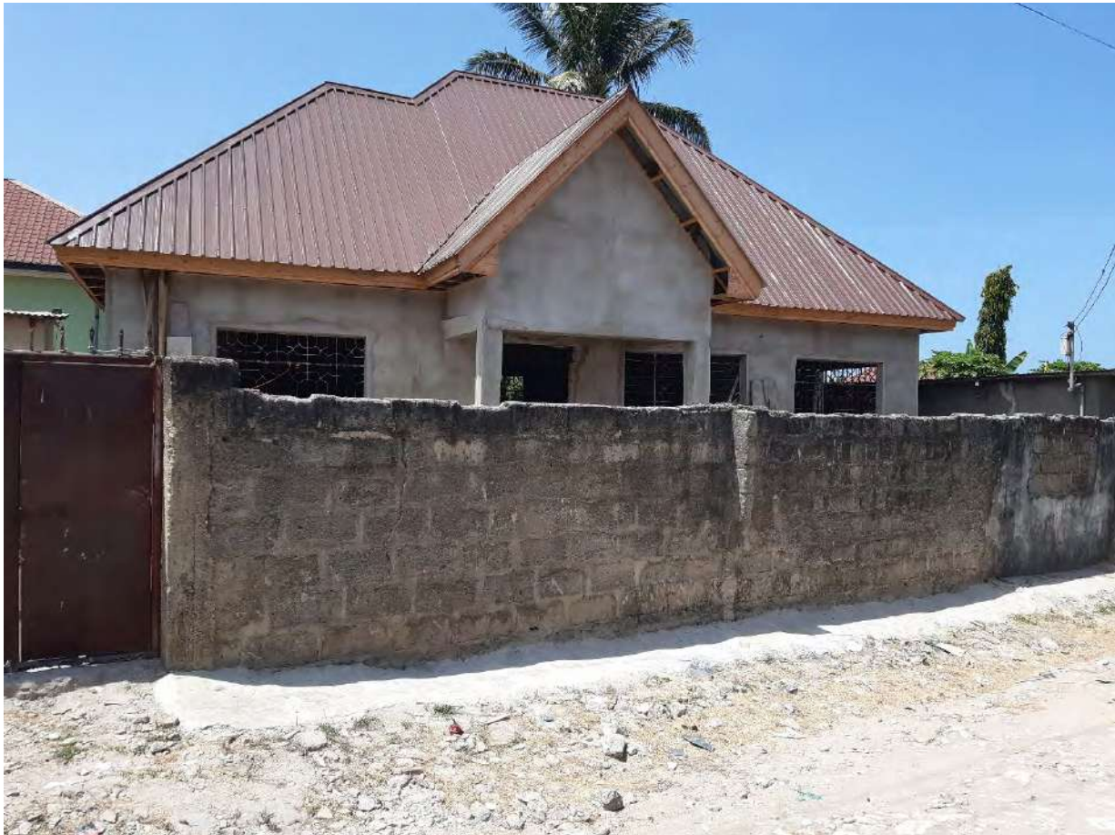
Fig. 2.4 - The figure shows repaired old buildings by extending the headroom and providing new roofing. Later the fence walls will be plastered by the owners. [source: Fieldwork, 2022]
